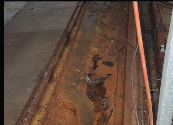
Fig. 2 Deteriorated air handler
