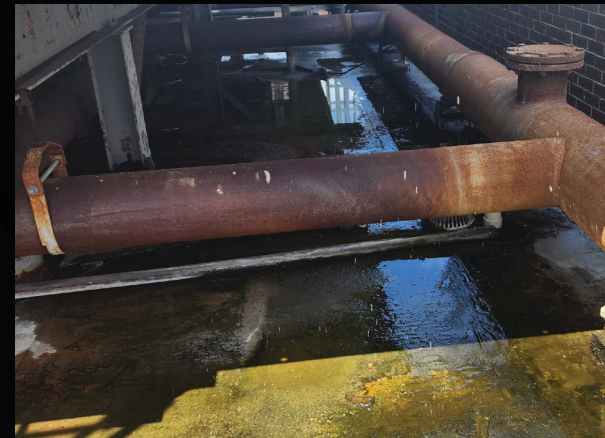
Fig. 1 Roof area below air handler
